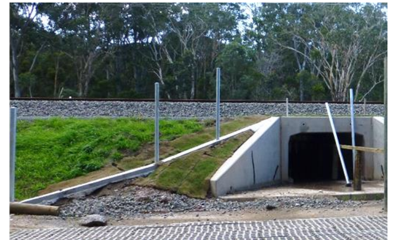
Figure 4.3.13. (photo D de Villiers) Koala exclusion fencing constructed along a rail line. Without barrier fencing, koalas will likely walk across the rail line and avoid the dedicated fauna crossing point/culvert. Fencing completed below.
