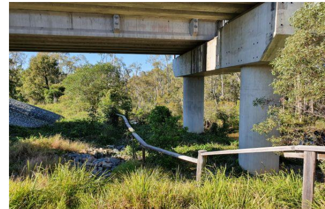
Figure 4.3.11 (photo D de Villiers) Under-bridge crossing point for wildlife, with wide buffer to bridge footings that can accommodate fauna furniture to assist with movements and predator avoidance.
