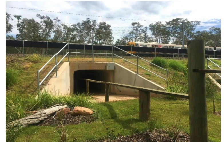
Figure 4.3.12. (photo D de Villiers) A 3.0 m x 3.0 m box culvert provides maximum light penetration and is large enough for fauna furniture to aid movement and predator avoidance.
