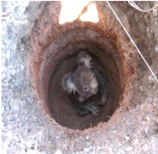
Figure 4.4.8. (photo D de Villiers) Deep post holes for koala proof fencing along a state road upgrade entrapped a koala that could not climb out of the hole.
